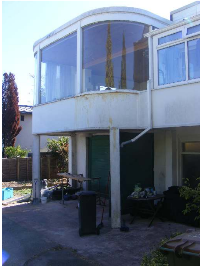
(02) Photo looking South-East at the existing projecting part curved bay window, serving the existing lounge, erected on pillars. In particular this photo highlights the canopy projection created by the bay window (proposed to be infilled), as well as the existing messy junction between the bay window and the adjacent conservatory structure.
